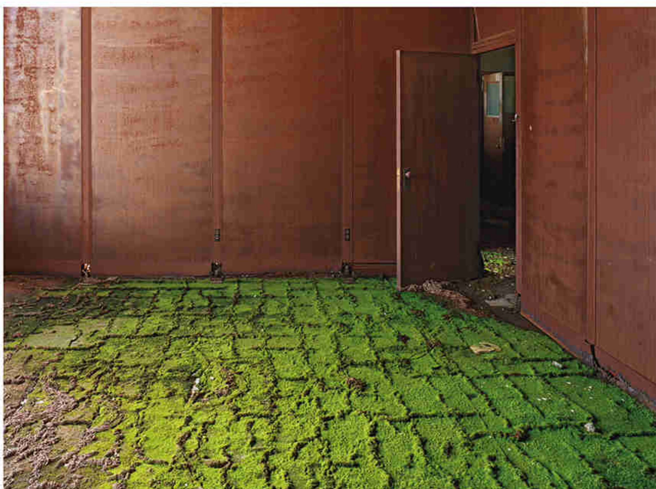
The Highland Park Ford plant was designed by Detroit architect Albert Kahn. It opened in 1910 and in 1913 became the first auto plant in the world to house an integrated, moving assembly line. Now it's a storage site, though some areas—like this moss-carpeted office in an administration building next to the factory—have been unused for decades.
